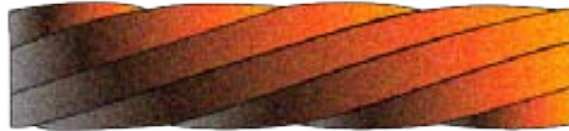
FIGURE 29 HEAVILY CORRODED ROPE
