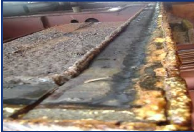
Worn rubber seal with evidence of foam
