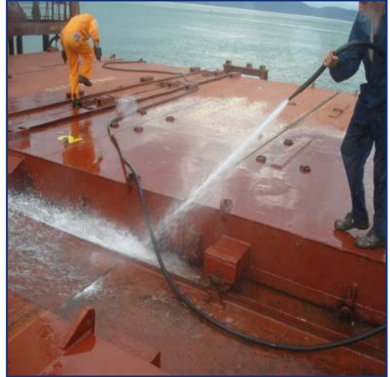
Jet Directed Incorrectly
