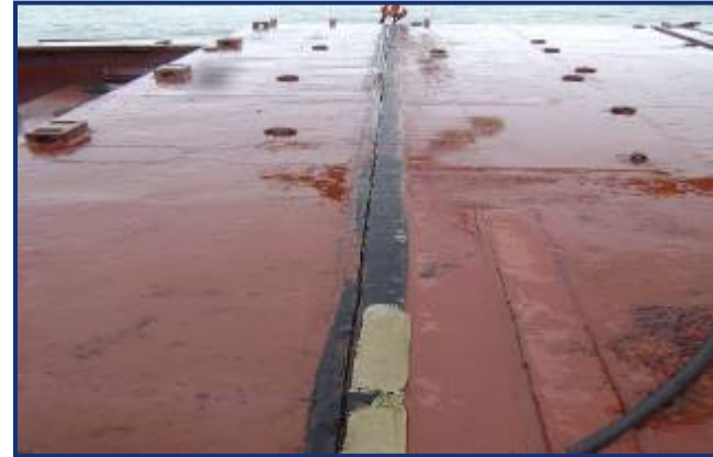
Evidence of tape used to seal cross joints
