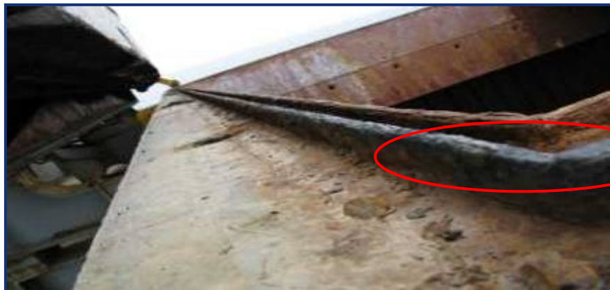
Compression bar wasted and pitted
