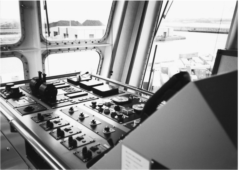
Remote controlling station. An enclosed bridge wing control station having dual controls for CPPs, bow thrust and numerous indicators for displaying operational data.
