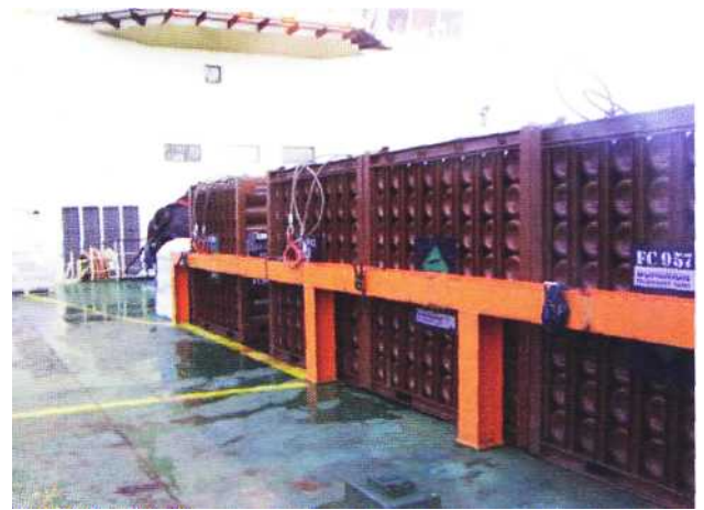
Figure 2.12 Storage of Gas Cylinders
