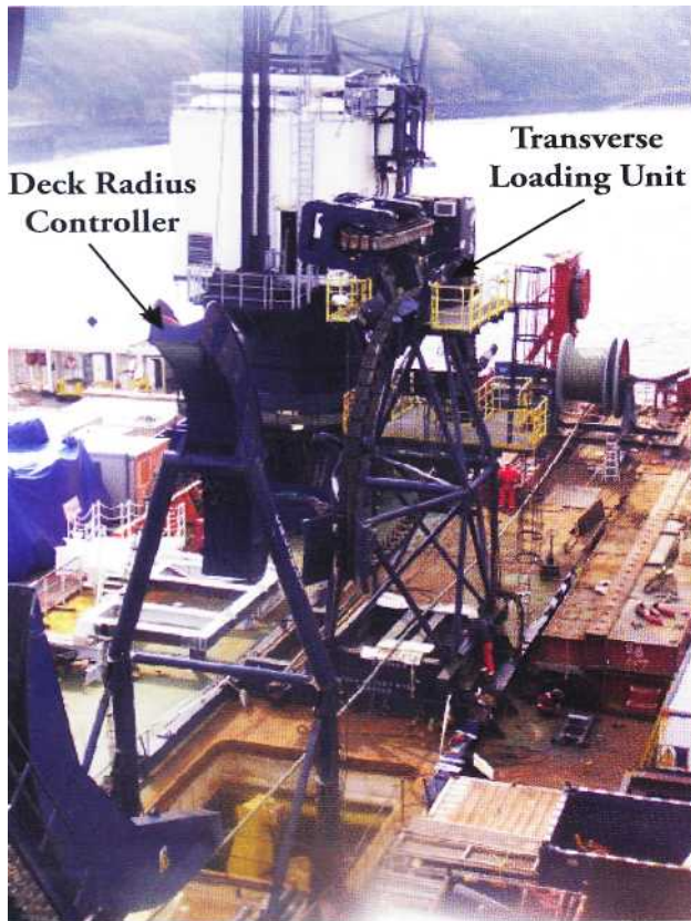
Figure 5.26 Loading Tower and Deck Radius Controller
