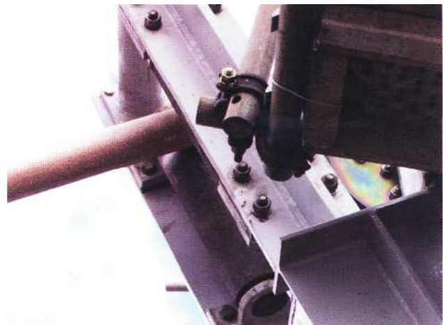
Figure 5-16 Exit Monitoring Frame
