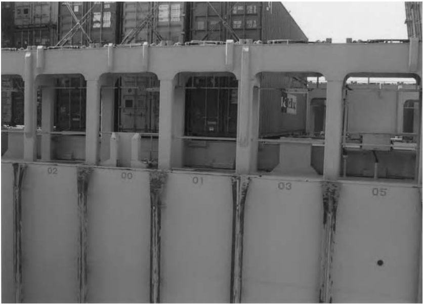
Fig. 8.1 Empty cell guides numbered odd to starboard and even to port, situated at the fore end of the cargo container hold.
