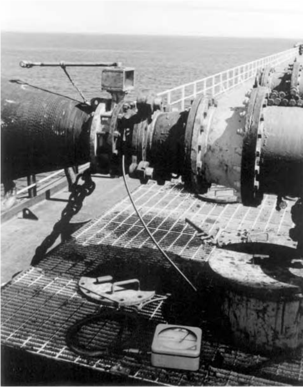
Fig. 5.11 Manifold and pipeline connections. Typical 14-inch oil pipe connection to the manifold.
