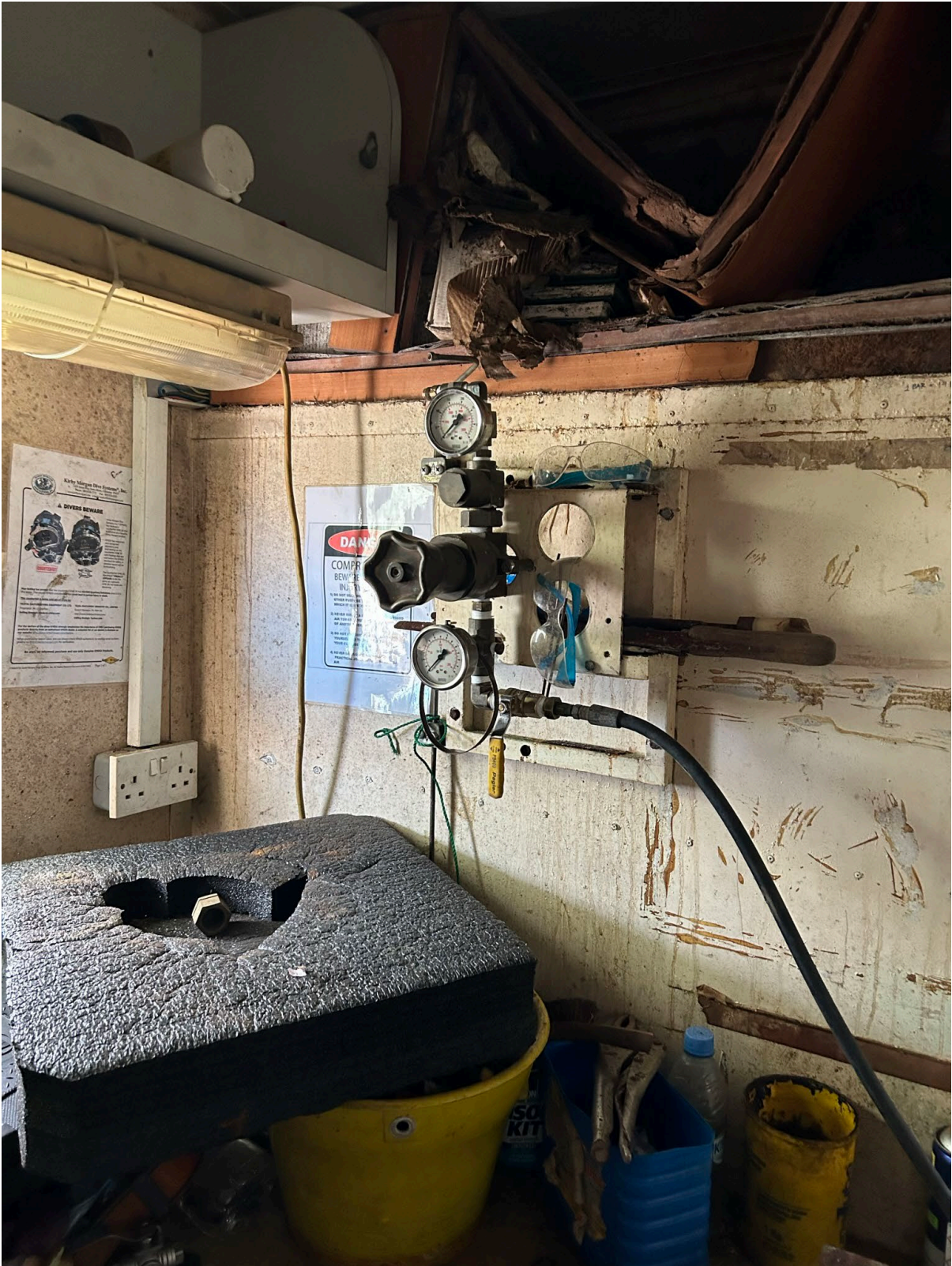
Compressed Air Panel
