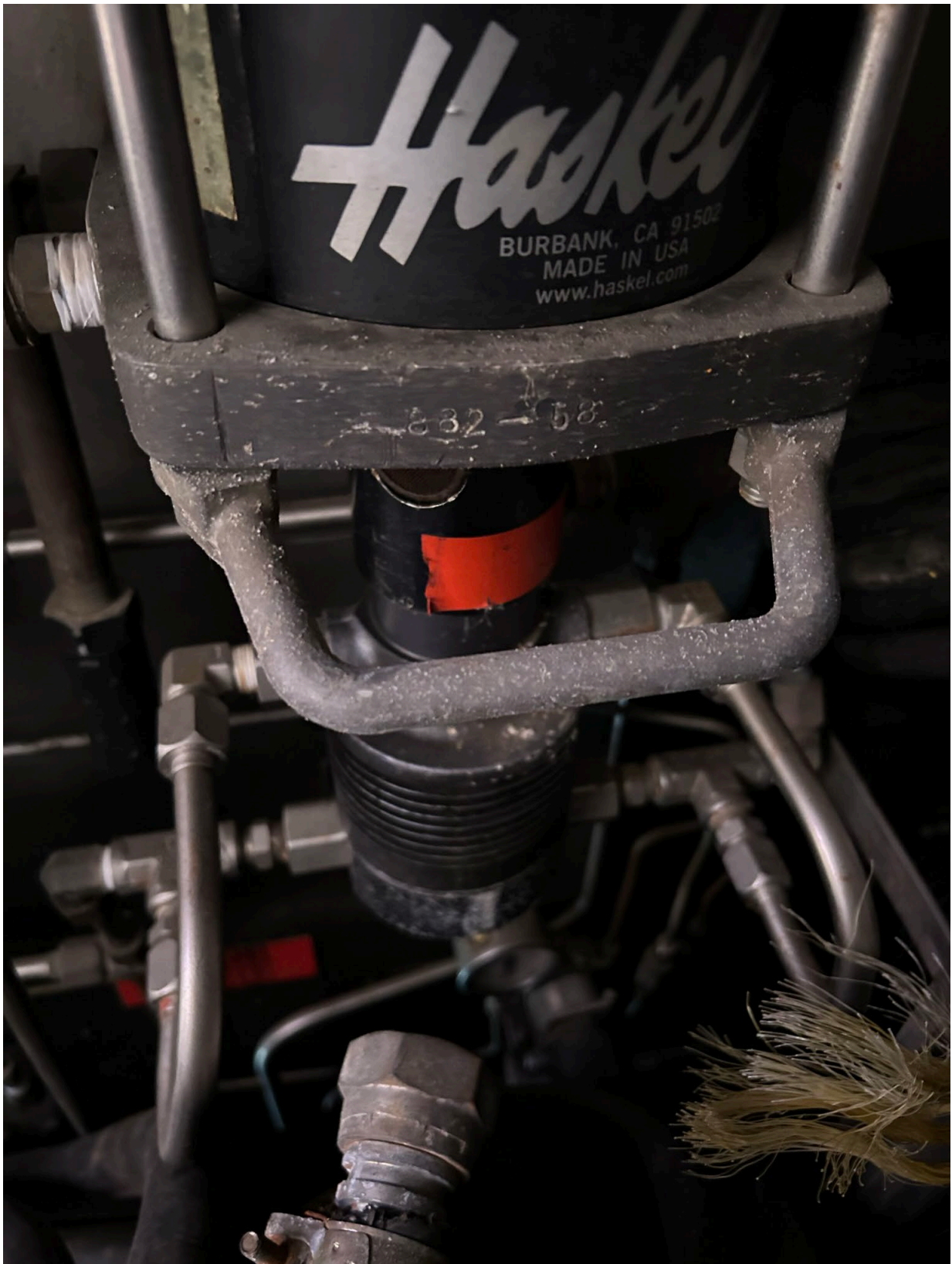
Haskel Pump on Gas Reclaim system
