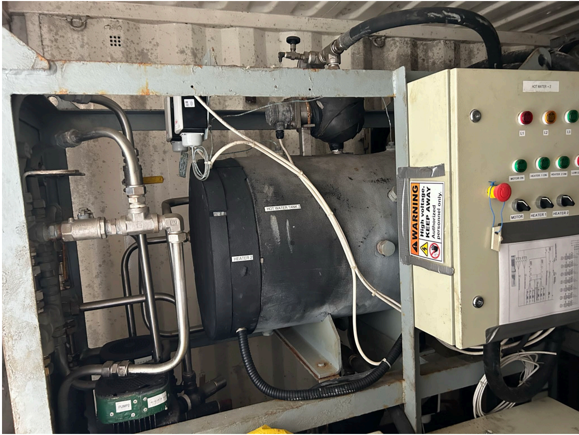
Hot Water Unit
