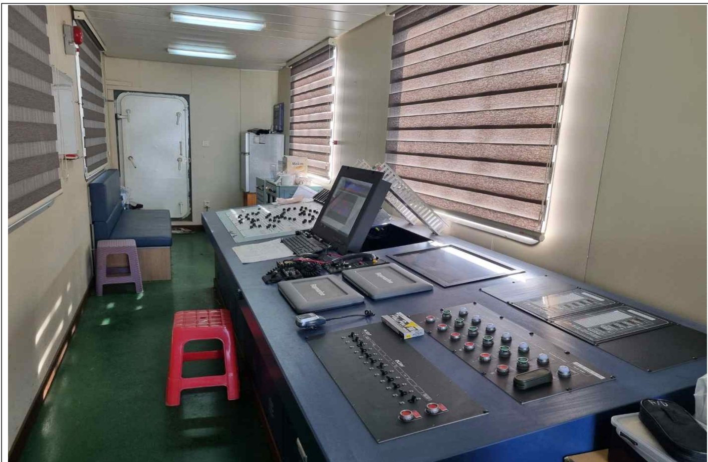
Ballast Control Room
