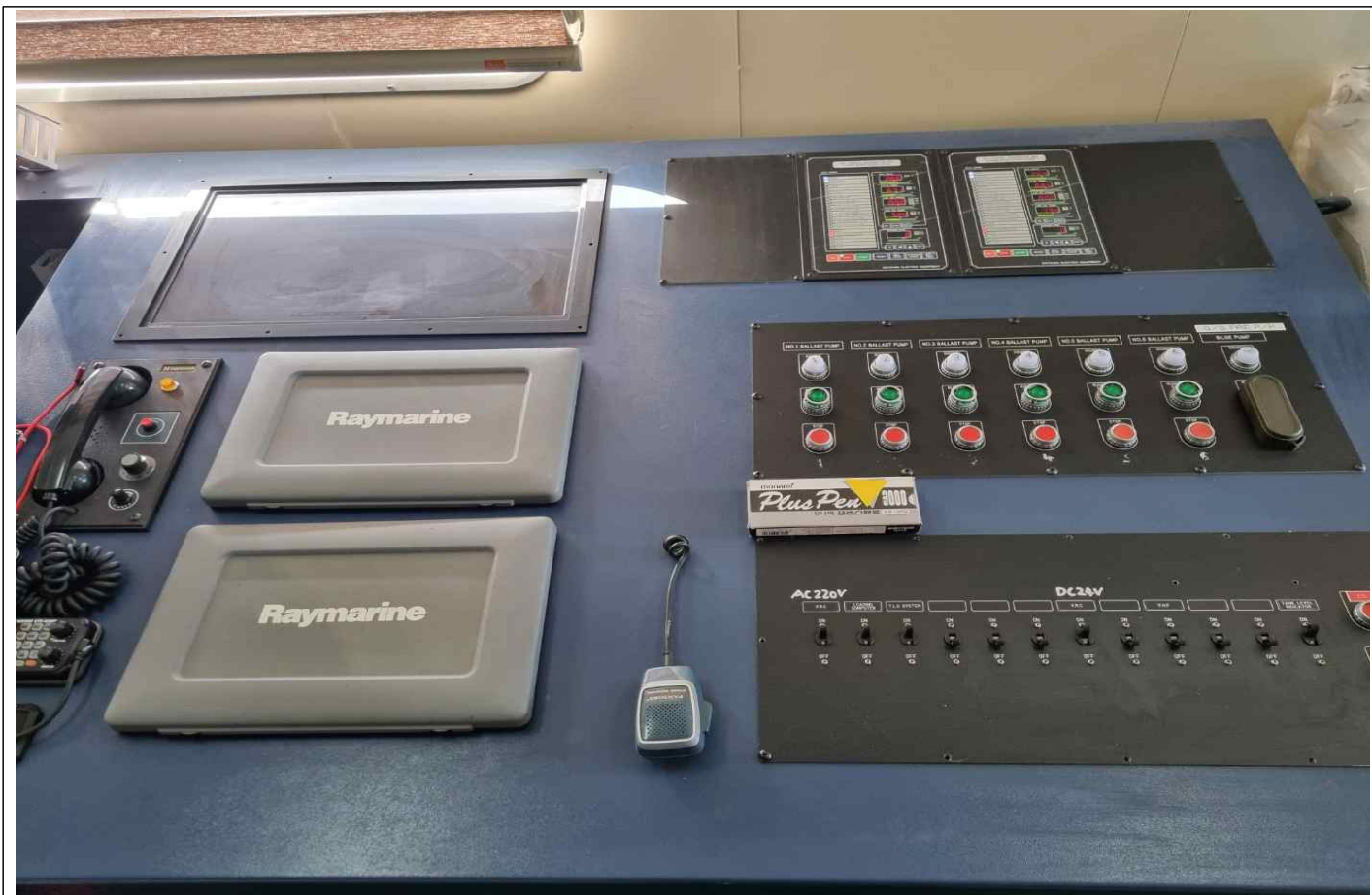
Pump ON/OFF Panel
