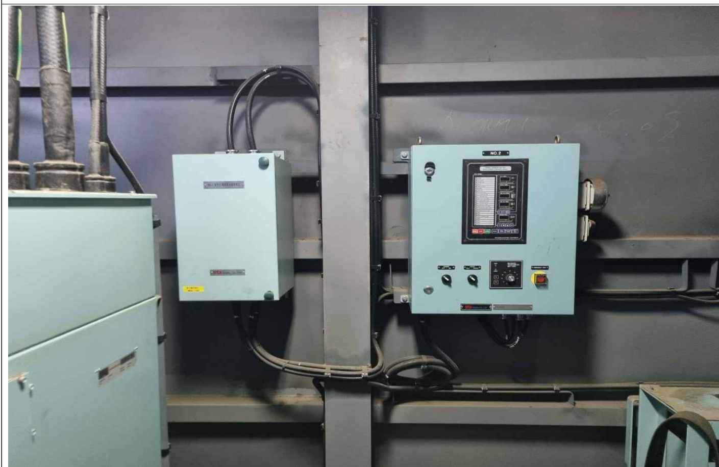
Local Generator Panel
