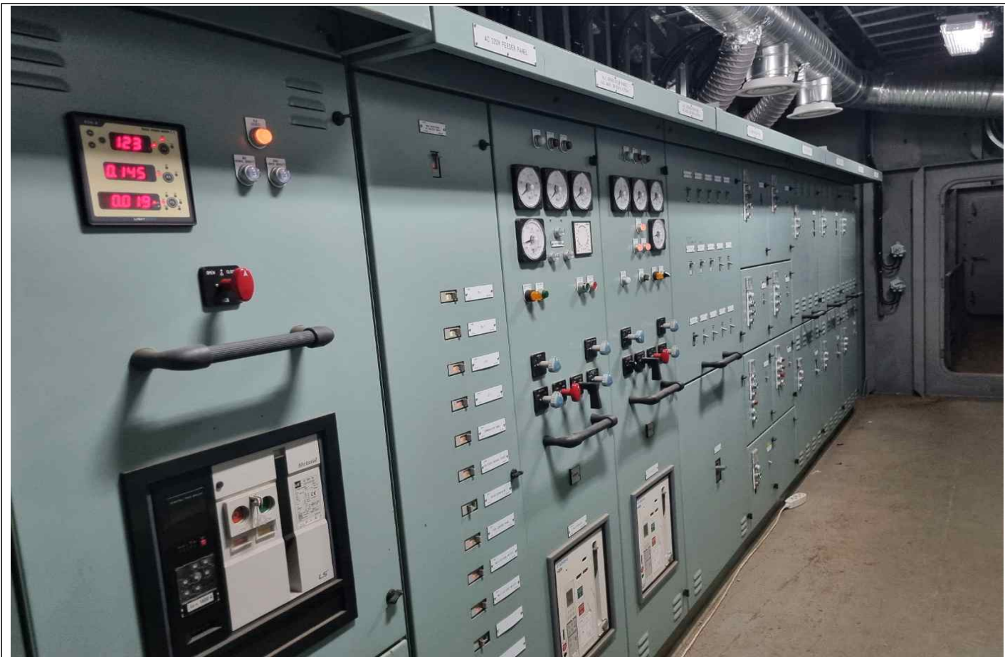
Main Switch Board Room (1)
