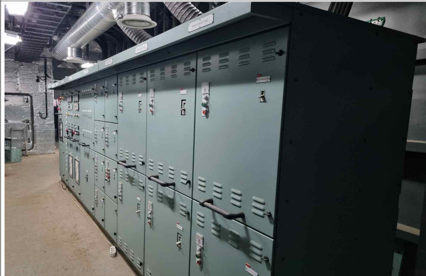
Main Switch Board Room (1)
