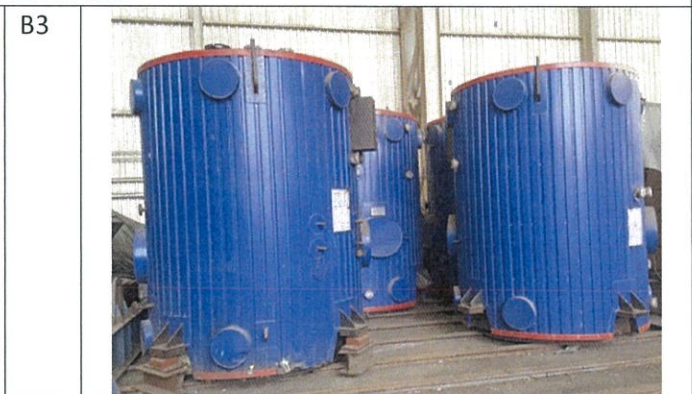
EXHAUST BOILERS: 4 (2 ENGINES PER SET) Vendor: AALBORG / ALFA-LAVAL
