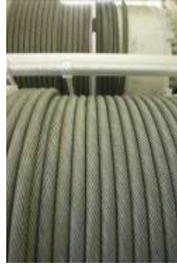
Figure 2: Winches inside crane house (typical)
