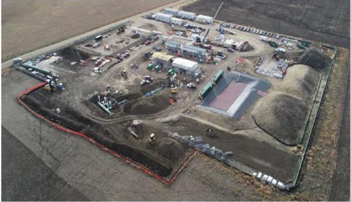
PUMP STATION 19 – October 2020
