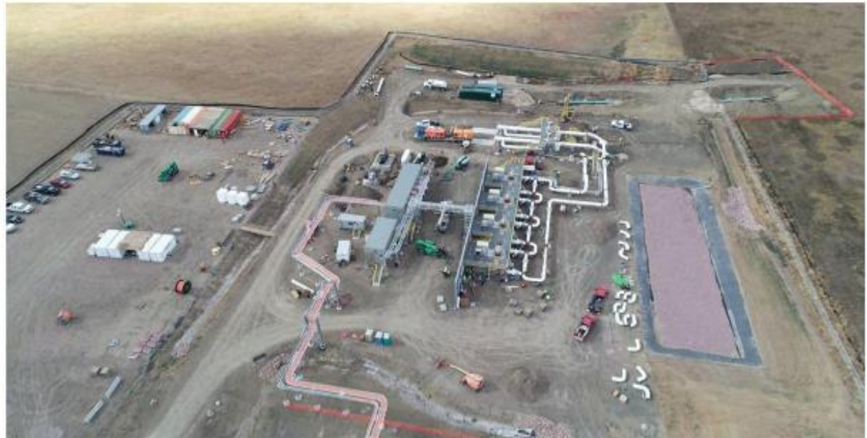
PUMP STATION 20 – October 2020
