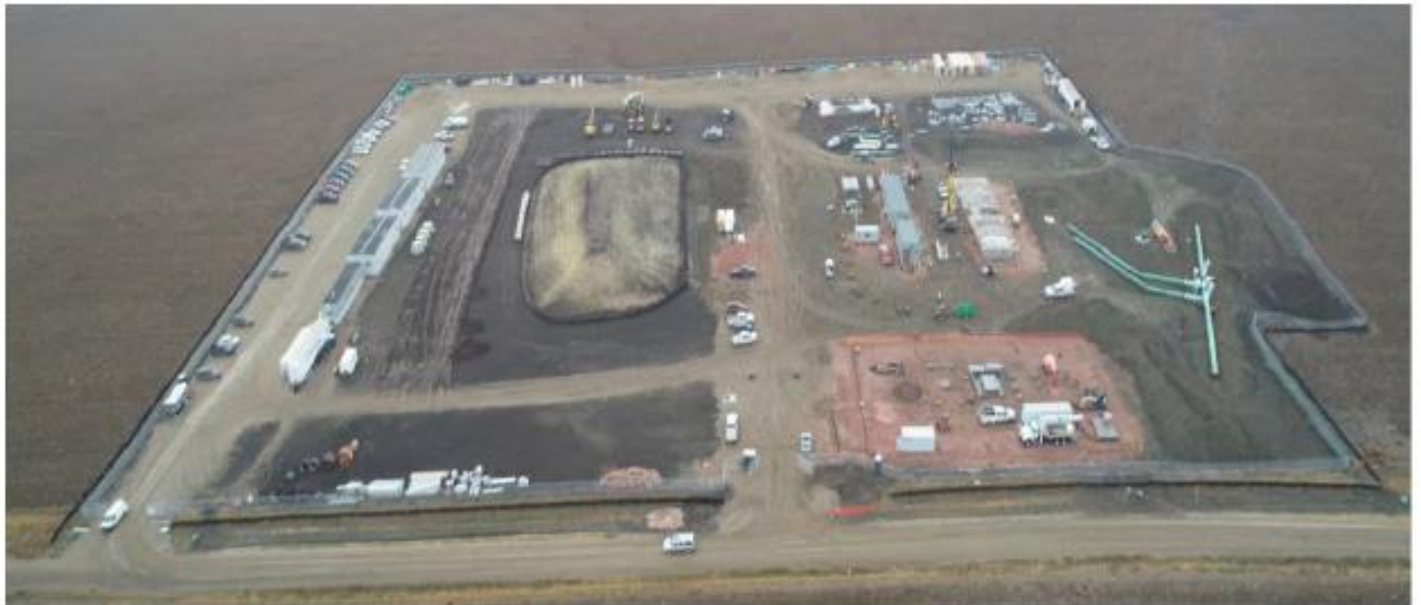
PUMP STATION 18 – October 2020
