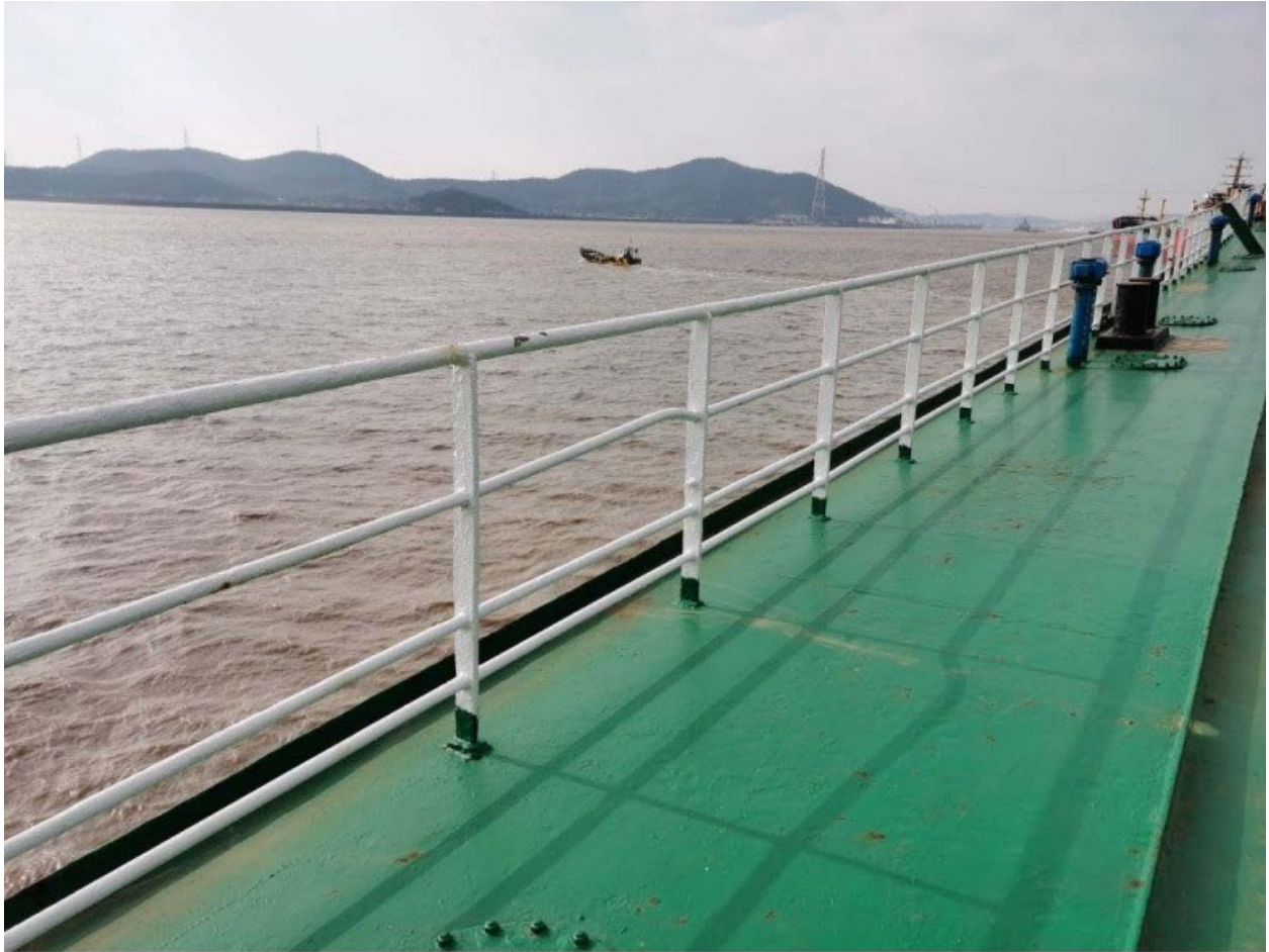
(27) Condition of main deck & guardrails
