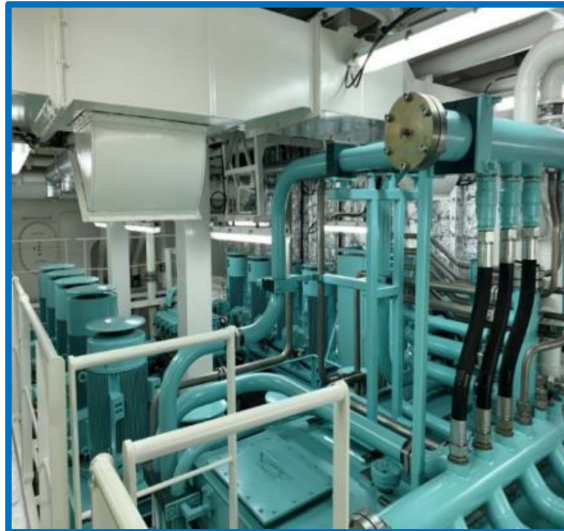
400T HPU Station
